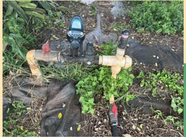
Riser Valve Connect to Sub-main (Photo: GoFarm Hawai'i)
